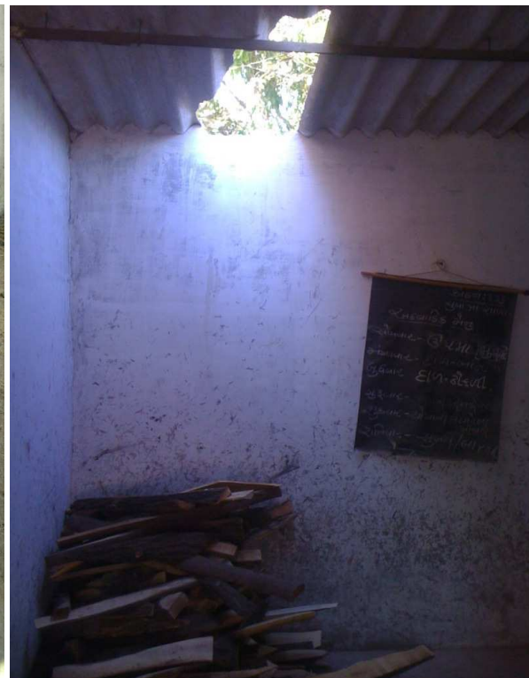
Kitchen shed needs to be repaired
