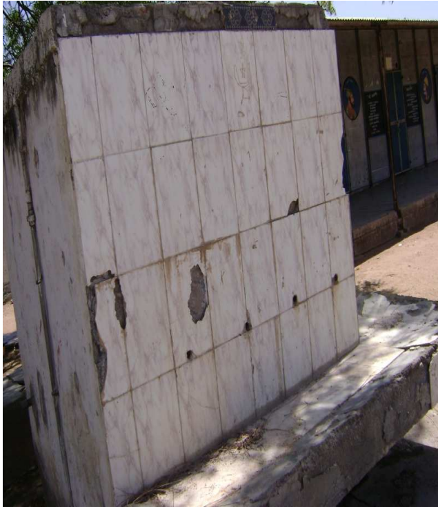
Drinking water tank needs to be repaired
