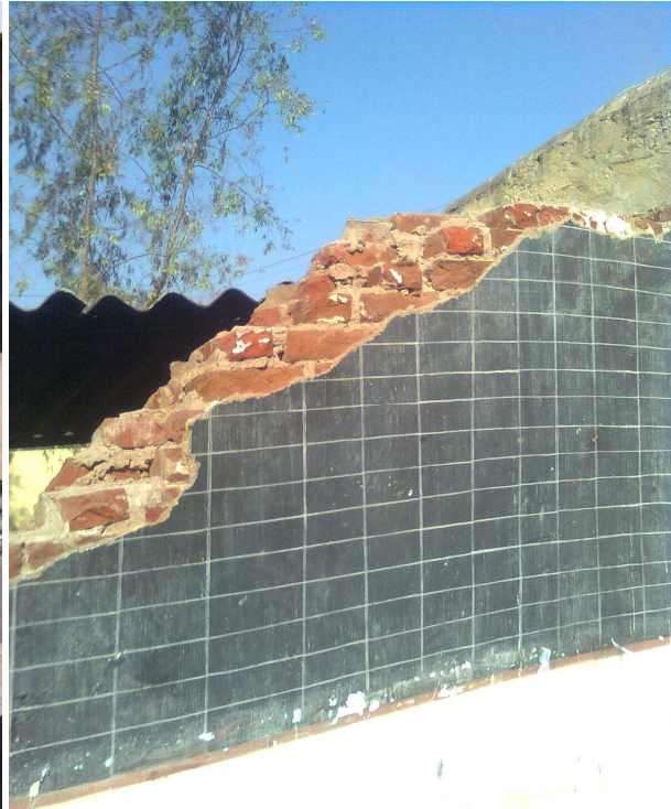
Broken wall of a kitchen shed
